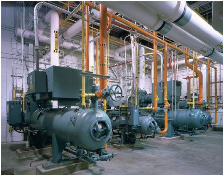
Compressors for large distributed system
