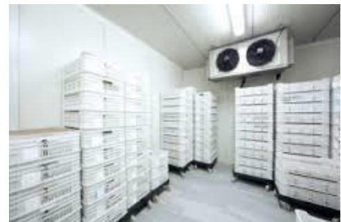
Small industrial system - evaporator in chill store
